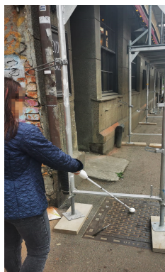
Fig. 4: A challenging situation when construction works happen in the middle of the pathway.
