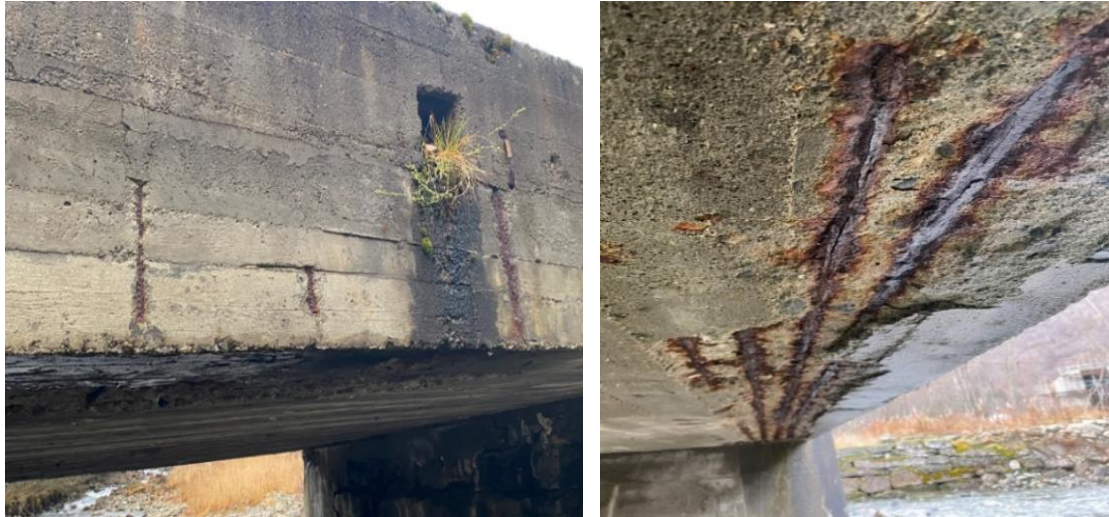
Figure 15: Spalling with exposed rebars on the sides & bottom of the bridge slabs
