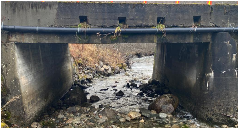
Figure 13: Efflorescence & small cracks detected on supports
