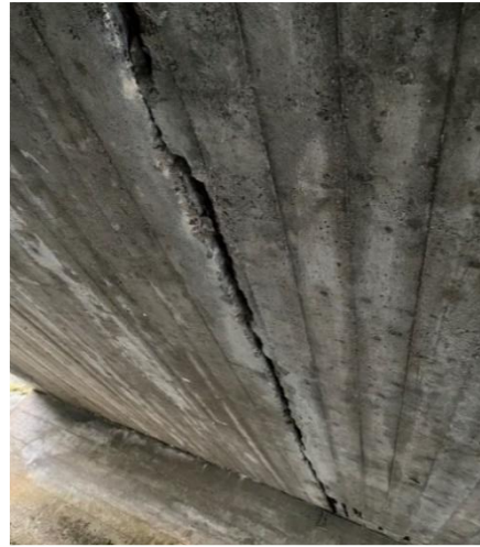
Figure 17: Longitudinal crack and spalling observed on slab A3
