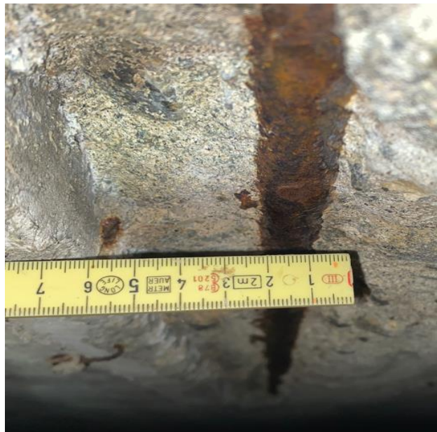
Figure 18: Longitudinal crack measured with exposing rebar
