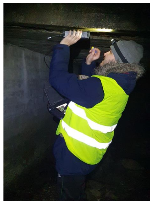
Figure 28: Profometer performed in situ
