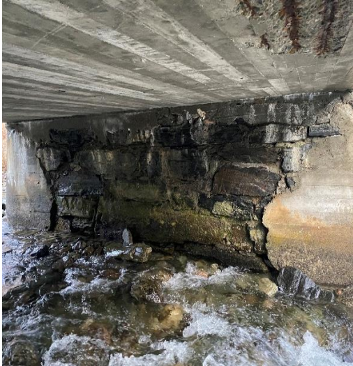
Figure 19: Potential erosion detected on support pier B2
