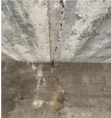
Figure 16: Efflorescence, plastic shear & longitudinal crack detected on A1 and B1
