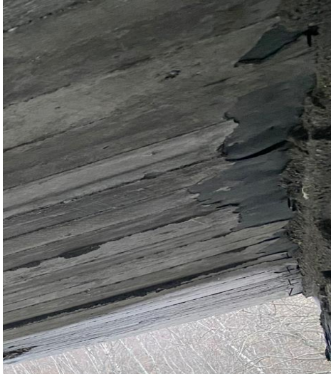
Figure 20: Delamination on the bottom of slab A2 on support pier B3
