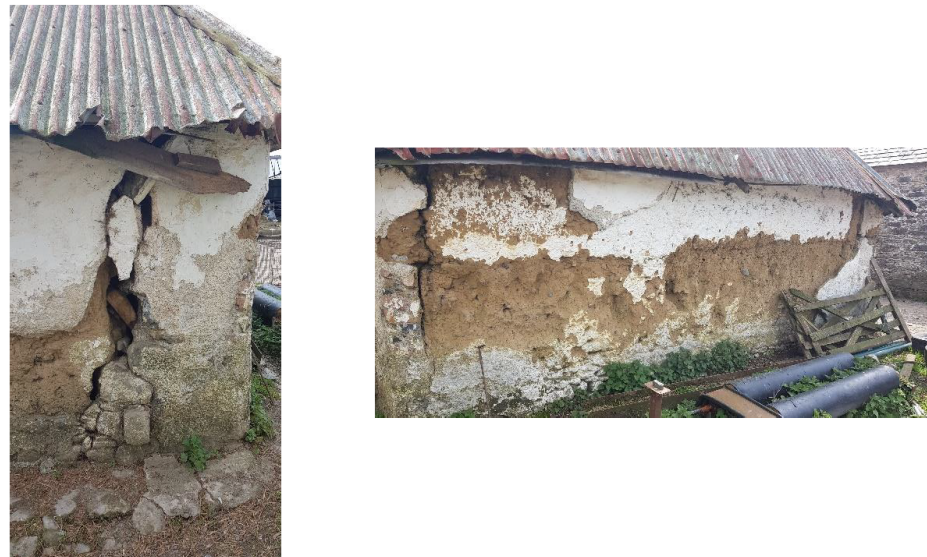
Figure 3. Vertical cracks in a cob building located in County Kildare, Ireland (pay special attention to the cracks at the corners running all along the wall's height).
