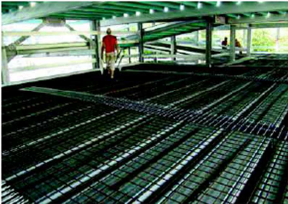
Multi-storey car park in the Gesundheitszentrum an der Nahe (health centre) in Bad Kreuznach
