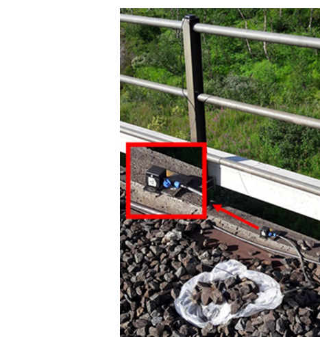
Fig. 2 Triaxial accelerometers on the bridge deck
