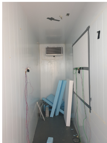
(a) Cold room
