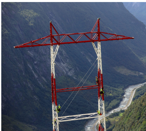
FIGURE 5.2. STATNETT'S H-PORTAL EXAMPLE [90] – 420kV SUSPENSION TOWER OF ØRSKOG - SOGNDAL POWER LINE. PRESENCE OF LINEMEN INDICATES THE SCALE OF CONSTRUCTION
