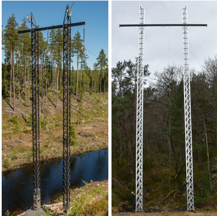
FIGURE 2.23. 132 kV ALUMINUM TRANSMISSION TOWER BY HYNDLA [81]. 18M H-PORTAL PYLON FOR RENEWAL OF LØVBERGSMOEN, LUTUFALLET AND TRYSIK TRANSMISSION LINE AND 21 M TOWER TEST PROJECT
