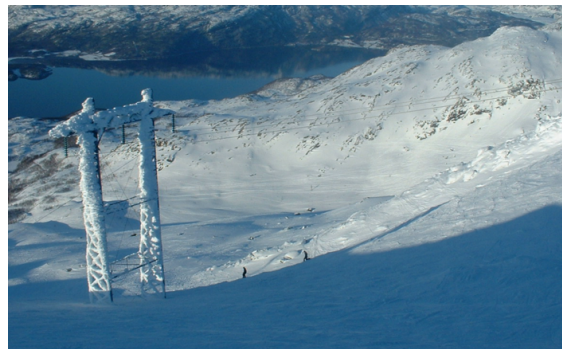
FIGURE 1.4. ICING ON 300kV POWERLINE IN NORWAY [16]
