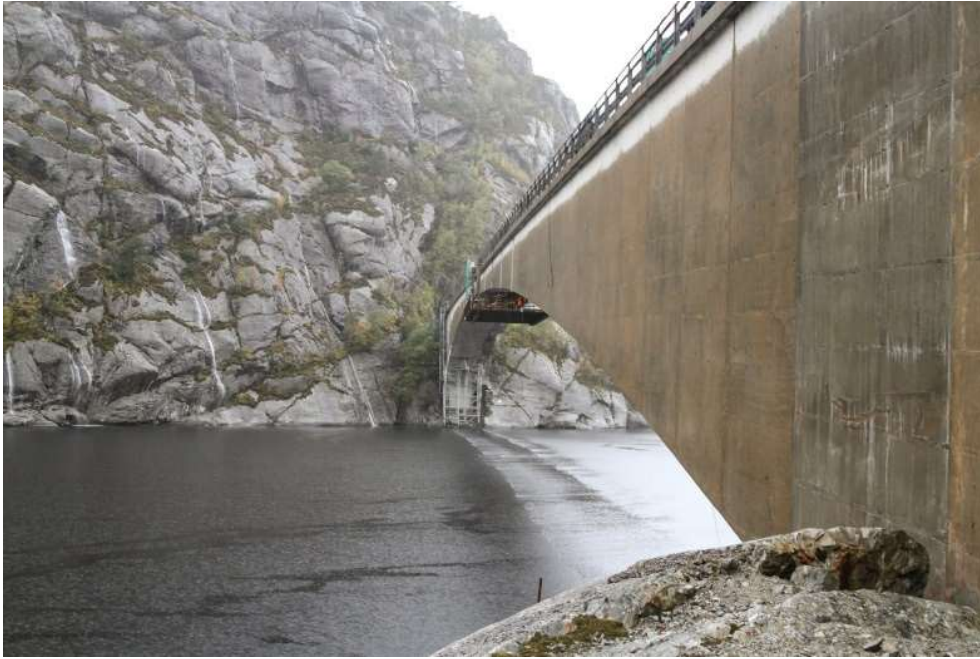
Figure 11: Bridge with added platform at the hinge where all the parts of the support system were inserted 5
