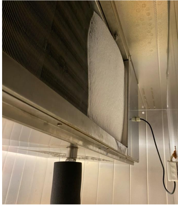
Figure 17: Ice growing on the cooling aggregate.
