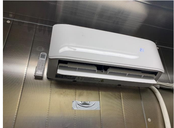
Figure 7: Heat pump on warm (red) side.
