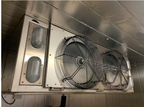
Figure 6: Cooling aggregate from inside of the climate chamber on cold (blue) side.
