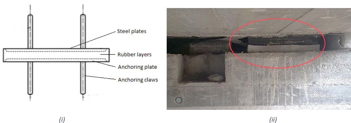
Figure 15. (i) Bearing ELASTO-BLOKK NBv [48]. (ii) Visual inspection of the bearing.
