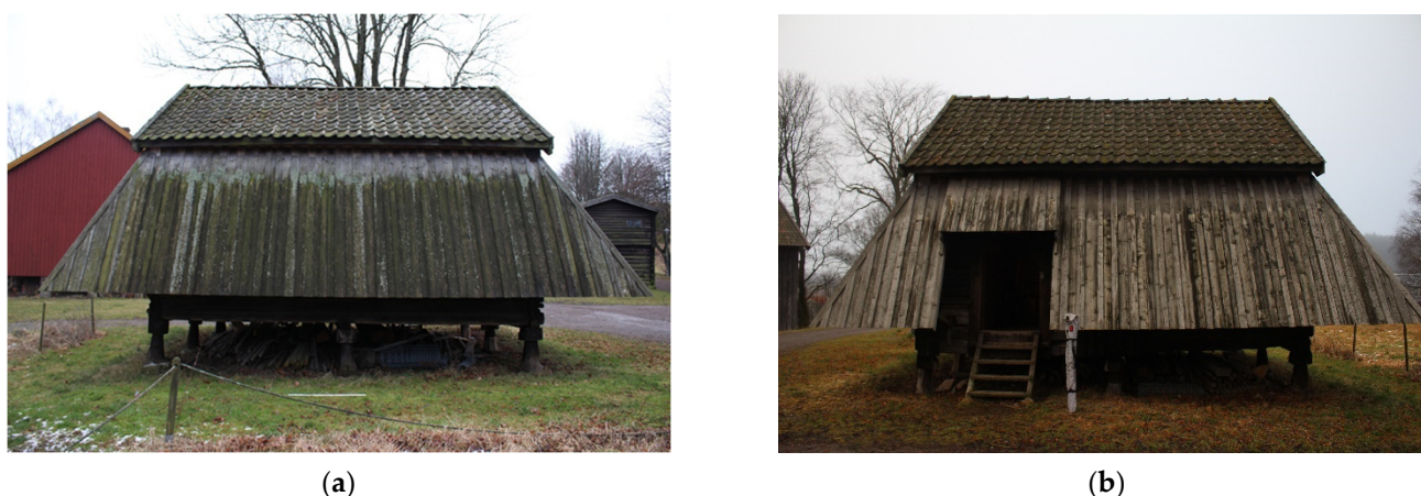
Figure 6. At the Fadum storehouse, the growth of biological organisms is more intense on (a) the north façade than on (b) the south façade.
