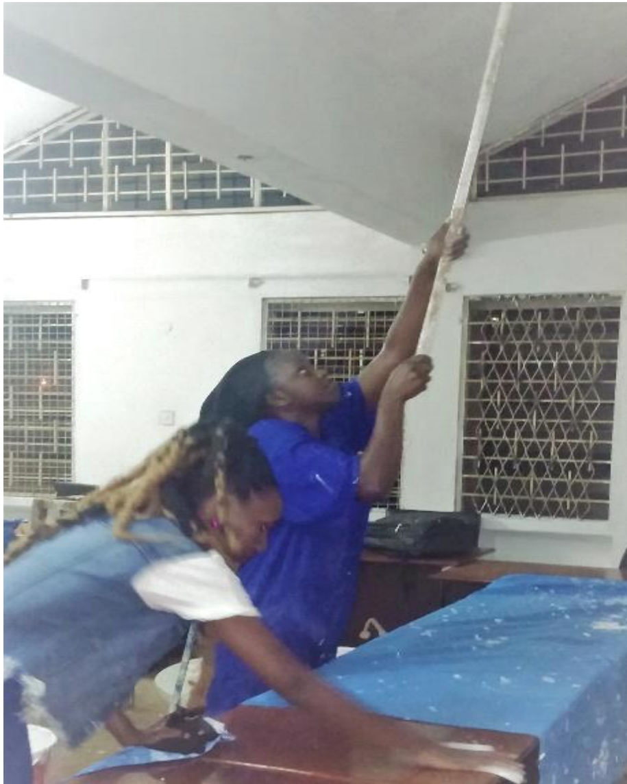
Figure: 4 Learners in a practical session, applying primer on the surfaces be application of the paint effects.
