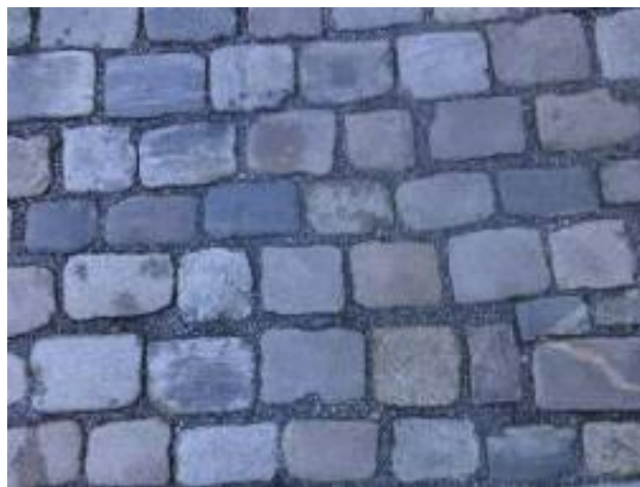
Figure 16: Permeable pavement at Bryggen (photo: F. Boogaard)
