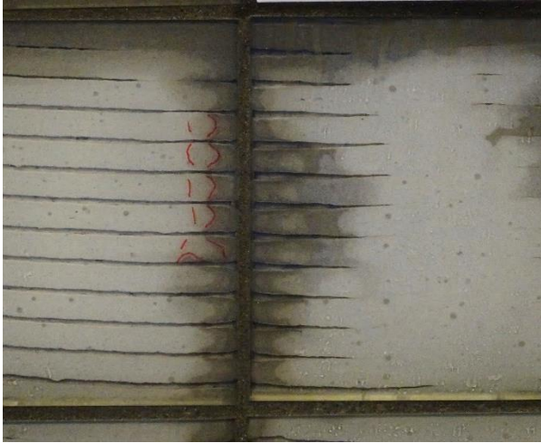
Figure 97 Moisture in Tile Adhesive where Moisture has Migrated from a Saturated Area to an Unsaturated Area through Diffusion
