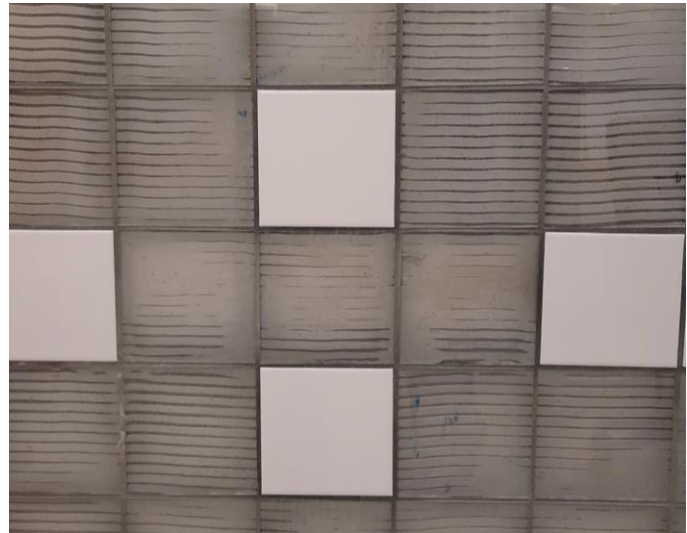
Figure 109 Wall #1 - Ceramic Tiles Functioning as Moisture Hubs Showing Moisture after 53 Days of Drying
