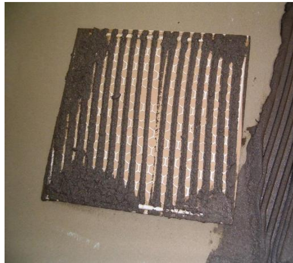
Figure 12 Visible Trowel Pattern in the Tile Adhesive due to Insufficient Tile Installation Pressure (II) - ref [56]
