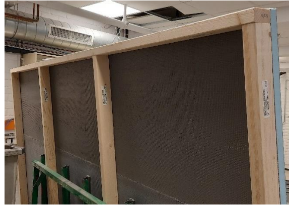
Figure 21 The Rear of the Base Wall Showing the Framework w/ Attached Litex Boards
