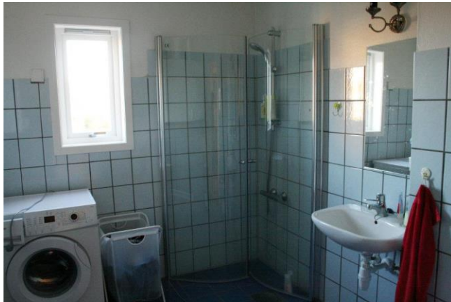
Figure 7 Glass Shower Door Installed on a Tiled Bathroom Wall [49]
