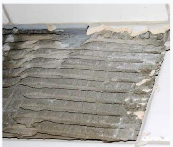
Figure 11 Visible Trowel Pattern in the Tile Adhesive due to Insufficient Tile Installation Pressure (I) - ref [52]
