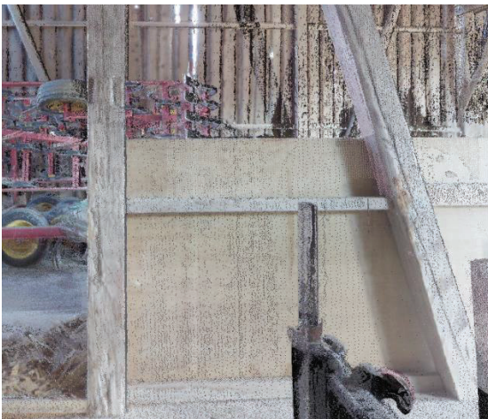
Figure 10. Screenshot from the point cloud of the barn showing damage.
