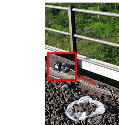
Fig. 2 Triaxial accelerometers on the bridge deck
