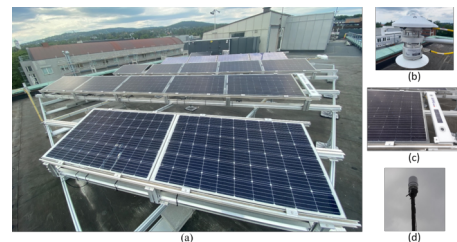
Figure 1: (a) PV demosite at SINTEF in Oslo, Norway; (b) CMP6 Pyranometer; (c) DustIQ Soiling Monitoring System; (d) Campbell Scientific CimaVUE 50 weather station.
