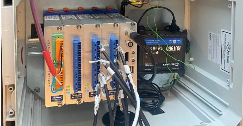
FIGURE 6: CONTROL UNIT AND DATA RECEIVING COMPONENTS INSIDE A PROTECTIVE CABINET
