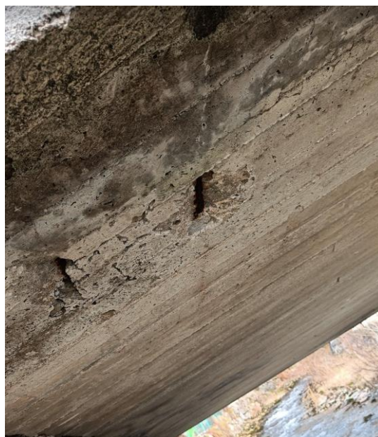
Figure 23 - Local concrete spalling where the reinforcement has started to corrode
