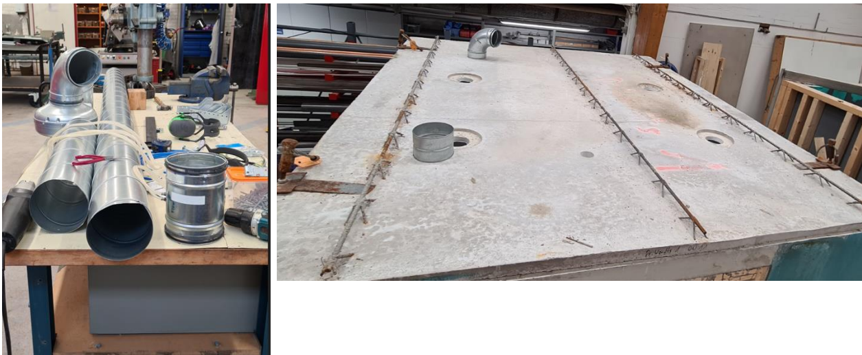
Figure 10: Setup for the ventilation and roof of the bathroom, image on the left figure shows the parts that were used to later connect on the roof of the bathroom module while image on the right shows the roof of the bathroom module before any ventilation exhaust was deployed.
