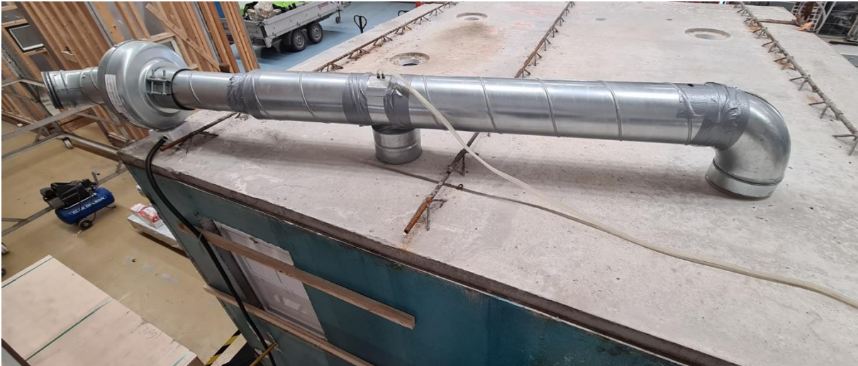
Figure 9: Ventilation on the roof placed over the shower
