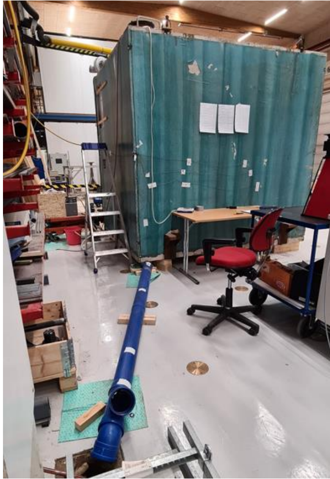
Figure 8: Drainage system, shower water returning from the bathroom
