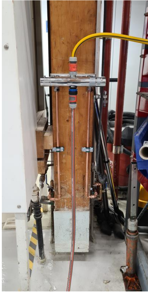
Figure 7: Mixer valve for adjusting the temperature for shower in the bathroom
