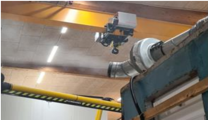
Figure 17: Ventilation exhaust, image captured when conducting smoke test for illustration
