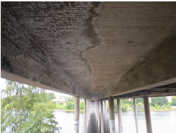
Fig. 12. Signs of water penetration of the bridge deck in outermost region of the bridge. Image courtesy of Dr. Ing. A. Aas-Jakobsen AS.
