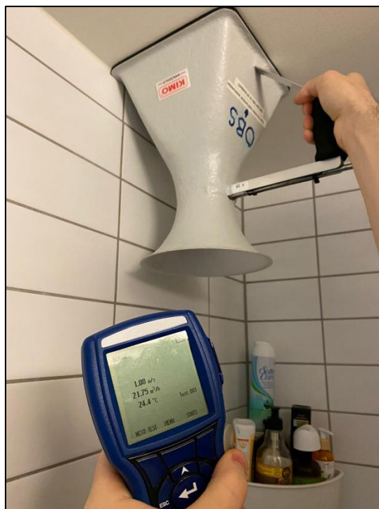
Figure 6. The measurement of supply air flow rates and mechanical extract ventilation air flows
