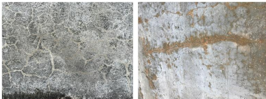
Figure 17 Map cracking due to ASR [23]
