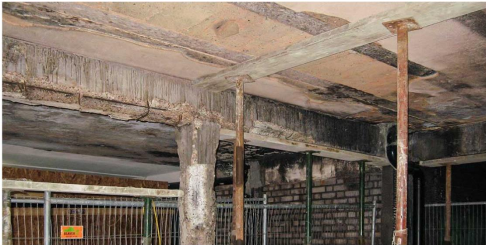
Figure 14 Spalling of concrete beam and column as a result of fire [31]
