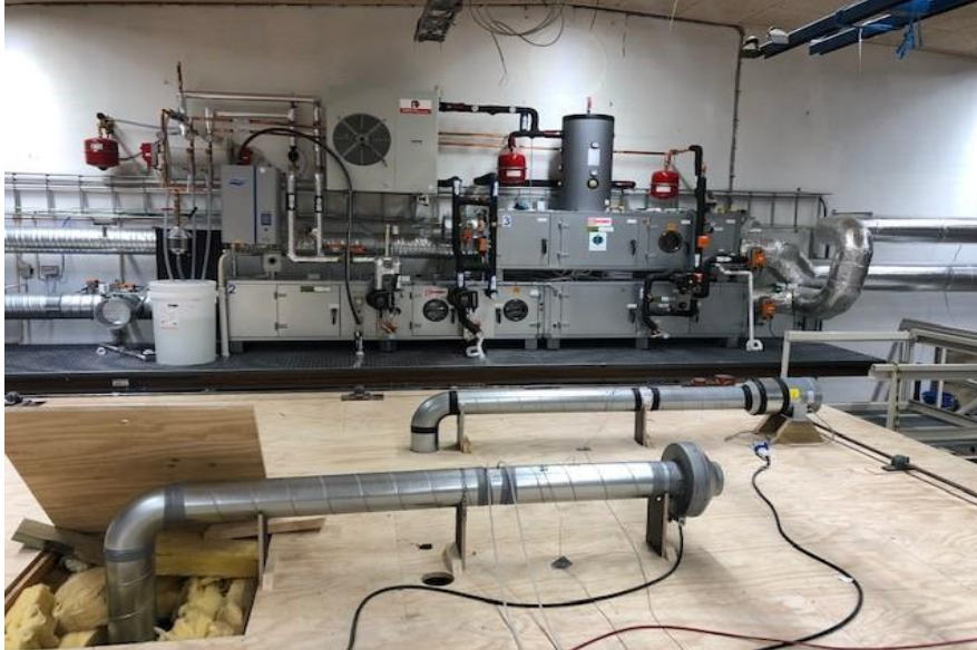
Figure 14: Installed AHU system
