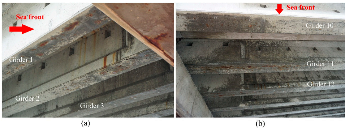
Figure 4. Corrosion-induced damage and humid areas in NIB girders: (a) in the first bridge span (1st to 3rd girders facing the sea) next to the middle support; (b) in the second bridge span (1st to 3rd girders facing the sea) next to the middle support.
