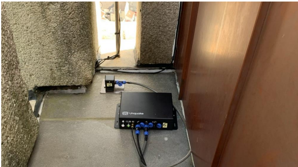
Figure 53 Sensor and datalogger roof - second reading
