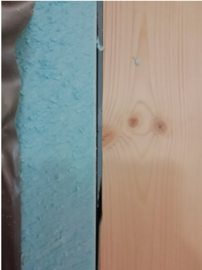
Figure 30: Unwanted gaps between the element and EPS due to poor manufacturing
