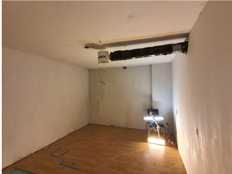
(a) PCM spackle applied to the inner surfaces of the climate room.
