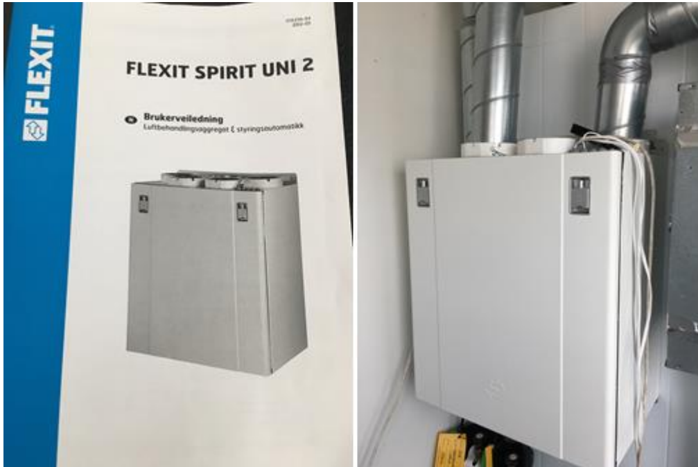
Figure 7: Pictures of the air handling unit connected to the study site of the PAQ study (Hangeland, 2018).
