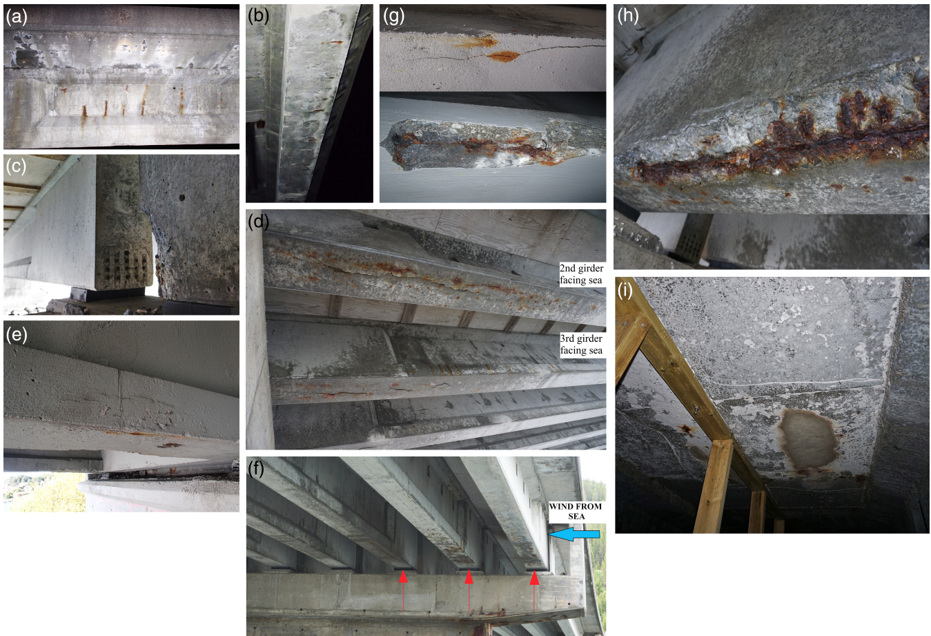
FIGURE 12 Typical visual corrosion damage in pretensioned NIB girders (a–i)
