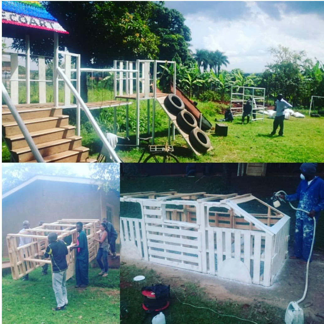
PICTURE 6: Construction of the different play elements on the site at KSPH
