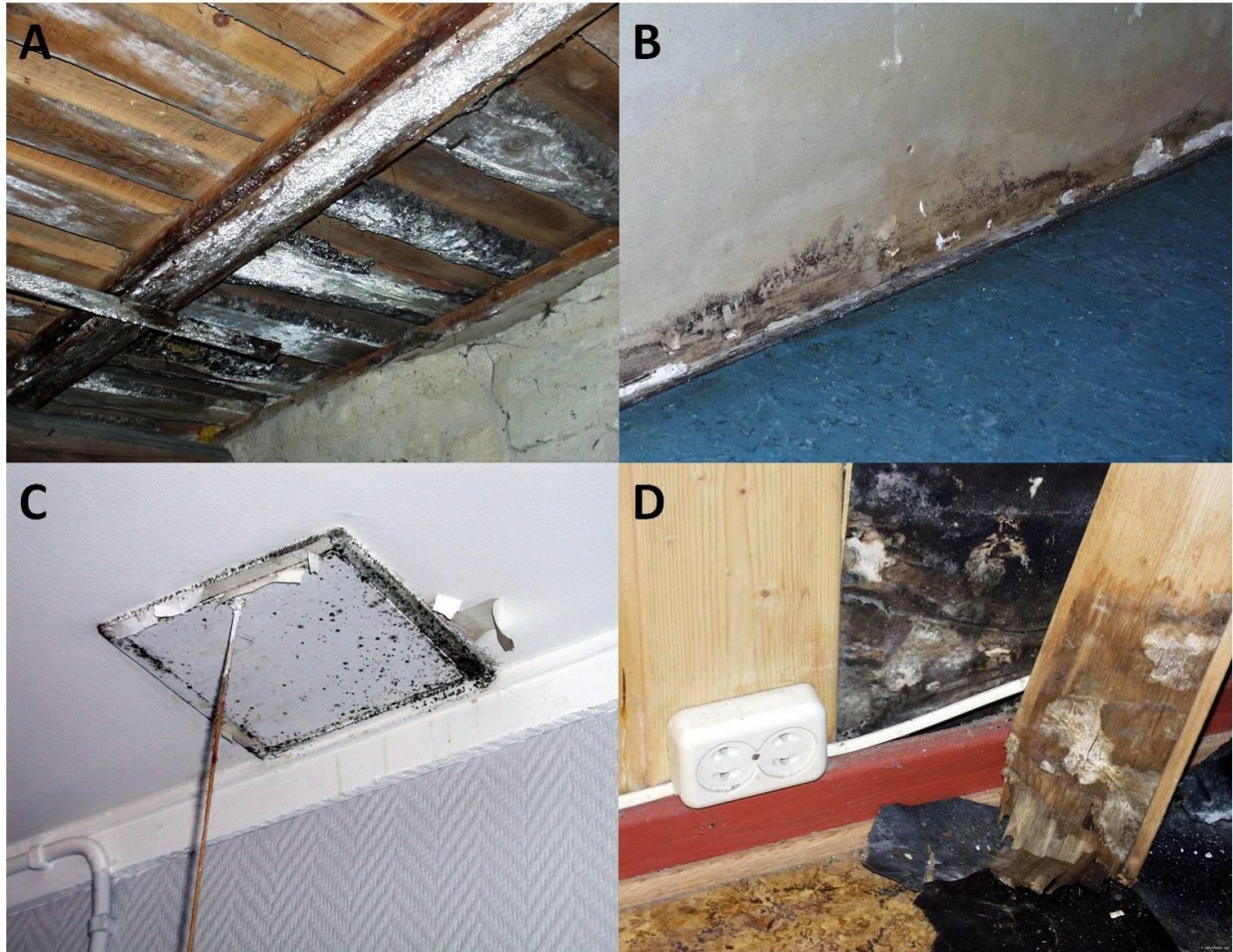
Figure 1. Examples of dampness related mold. A: Mold on roof beams due to condensation, B: Mold behind a skirting board, C: Mold infestation on a roof hatch due to condensation, D: Mold infestation behind wallboards in basement. All photos are courtesy of Mycoteam. Photos are obtained from www.mycoteam.no/bilder/#1 .
